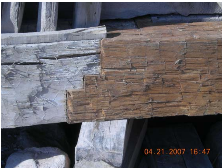
Base Timber, south wall, fitted to a second base timber. Both timbers are about 25 feet long and weigh about 2500 pounds of red oak.
